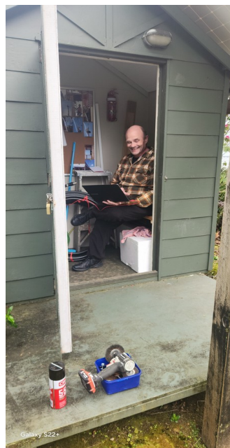
Greg ZL2BZH new repeater install
