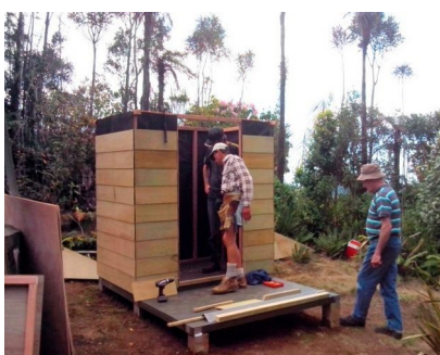
The Hut goes onto the floor with the help of Colin ZL2AHY and Peter ZL2APJ (SK)
